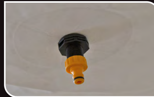
Central Drainage Point
